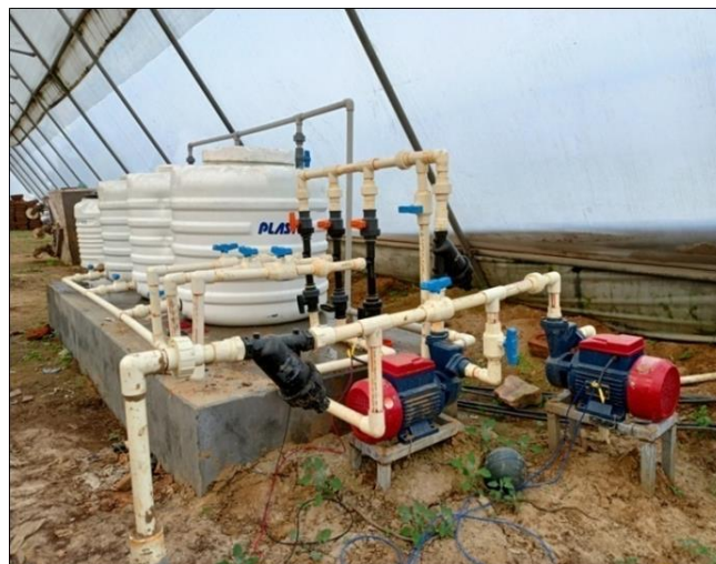
Fig. 6. Field view of developed fertigation control head
