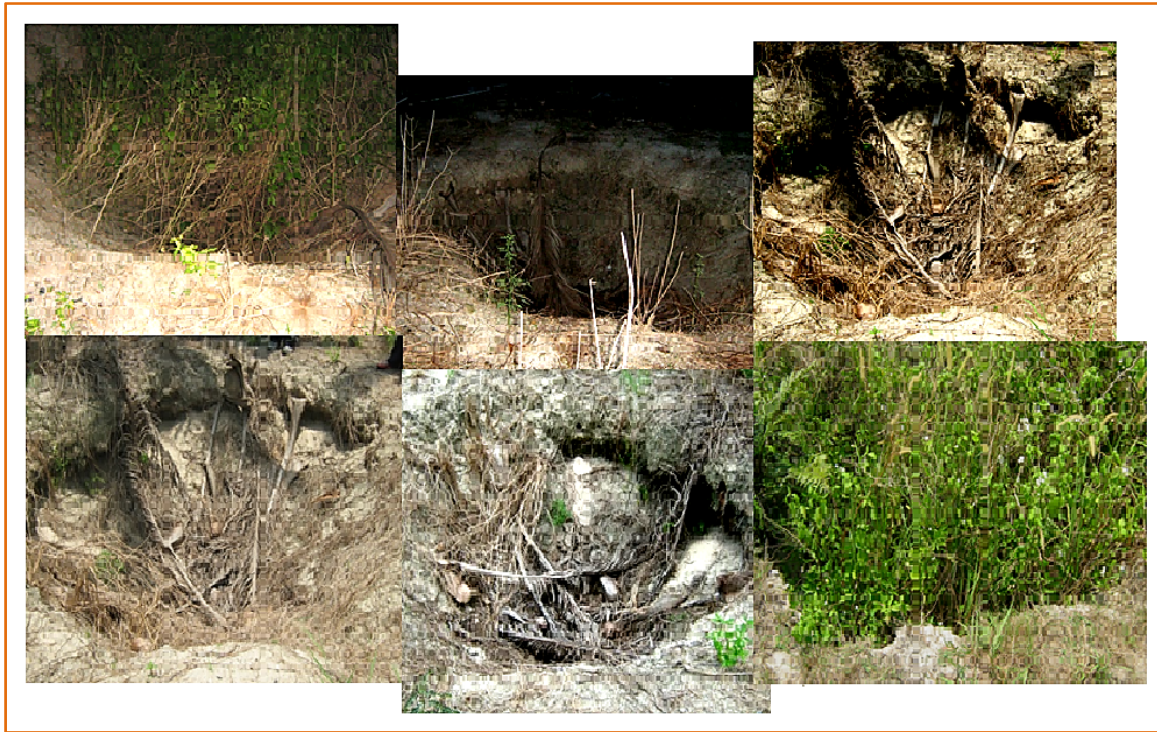
Figure 16. Several of small sinkholes describe as empty, sand in-fills and crammed with vegetations were identified during the site ground work inspection
